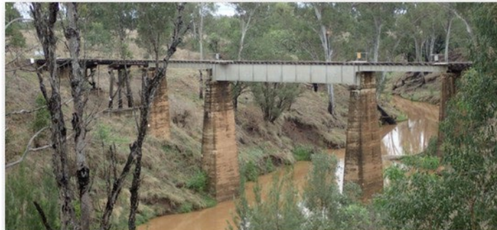
Many of the bridges traverse steep and deep creek valleys. Retention of the bridges is far preferable to construction of a lower level crossing.
